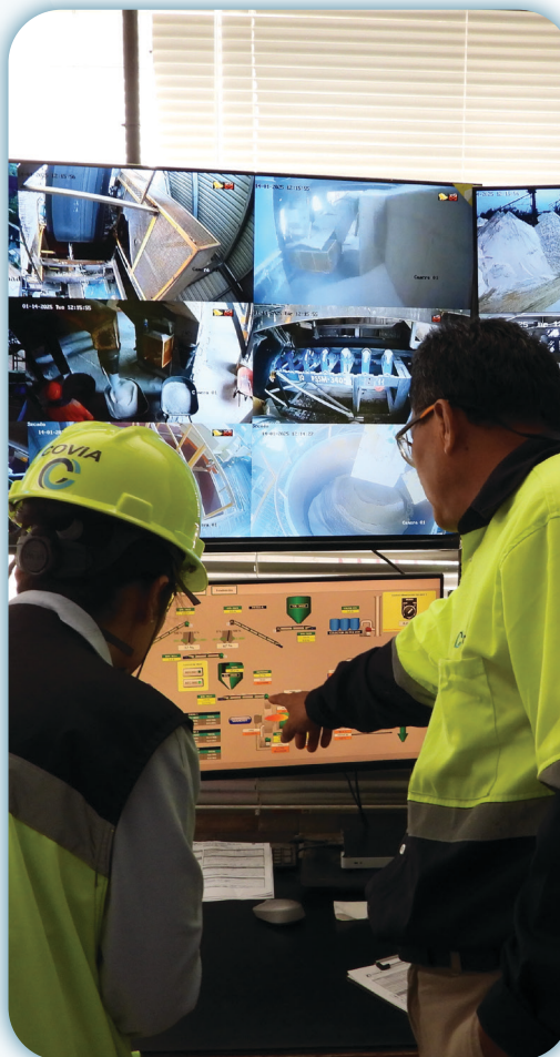
The Control Room (Ruben Peña)
